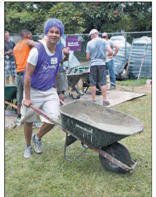
Joe Peach Graves (in KaBOOM! purple wig) with cement ready to fill the hole for the rocket ship. Photos by Rachel Breit, rbreit@midweek.com.
