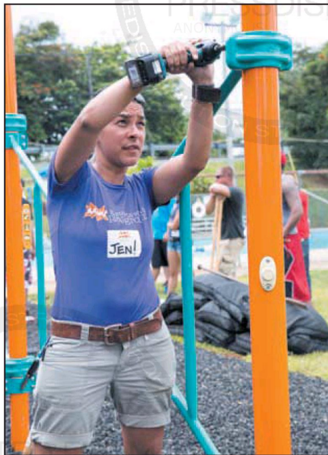
Jen Leshnowar, a KaBOOM! project manager, tightens some screws at the structure nears completion.
